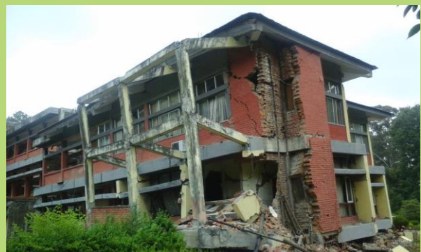
Damage to Tribhuvan University caused by earthquake
